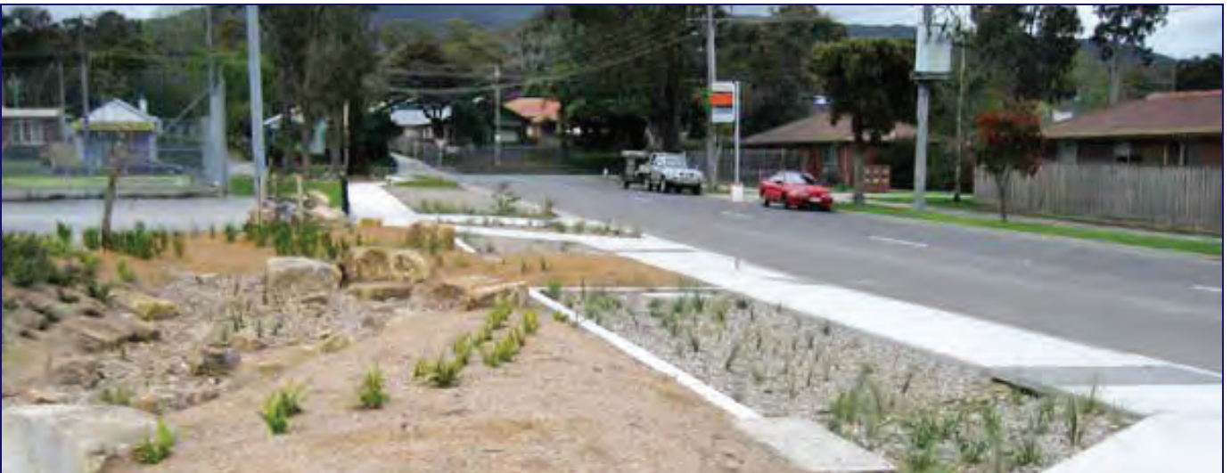
Recent street projects in Knox have used water sensitive urban design to improve water quality in Knox's waterways. Photograph in Boronia
