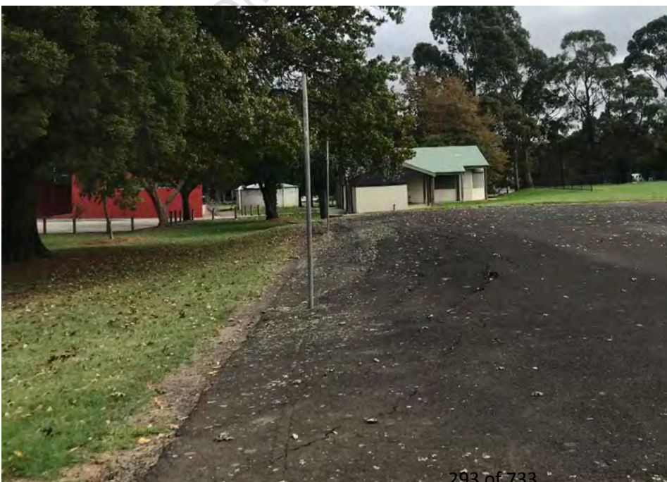
The court surface has deteriorated at the southern end, and is unsuitable for use in its current condition.
