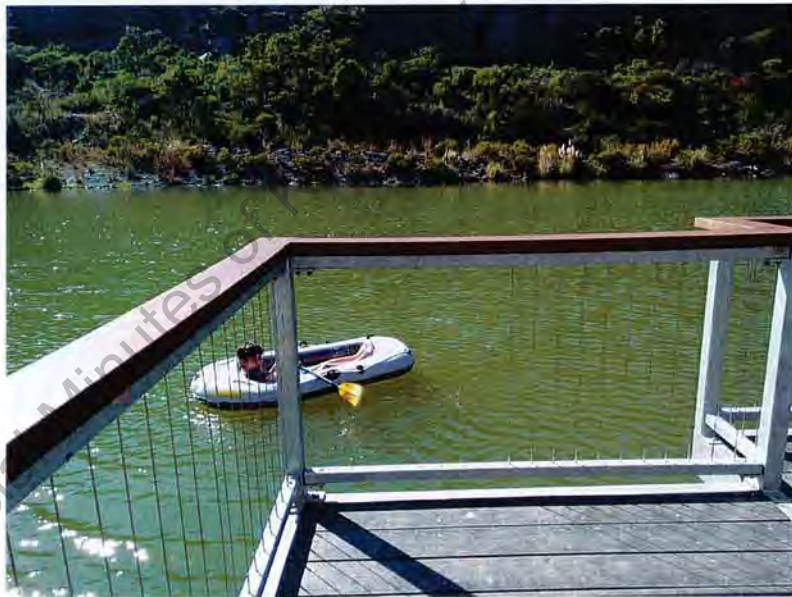
Photo 3.3: Fence cut out on Jetty (March 2017)
