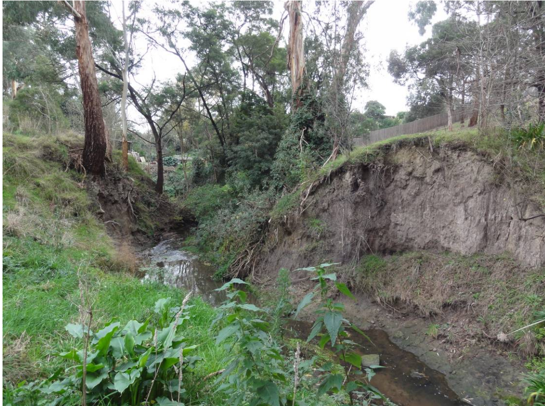
Figure 6. A representative scene within the creek channel, showing the water, an inclined bank apparently created by heavy machinery (bottom left) and steep, eroding banks with variable vegetation.
